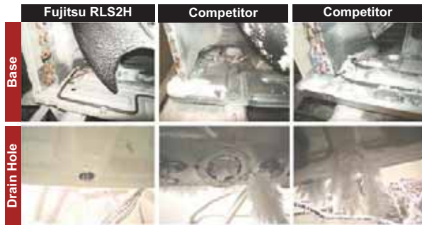
Drain hole is not filled, no freezing of base | Freezing where there is no heater | Drain hole is closed, large freezing of base
